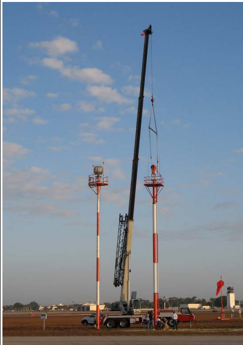
A new rotating beacon and tower being installed recently at Page Field.
