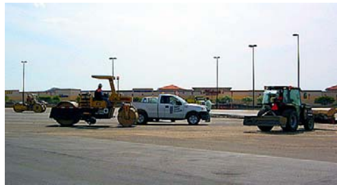
Paving of the new terminal ramp at Page Field is nearly finished
